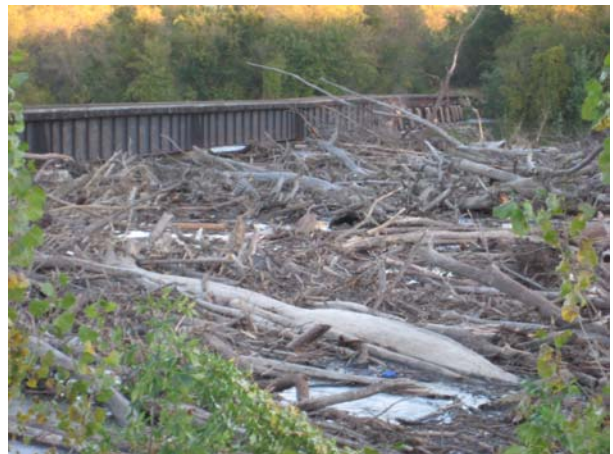
This is a log jam at the Carver Bridge.
